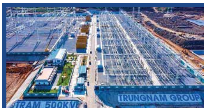
Trung Nam Solar Power Plant
